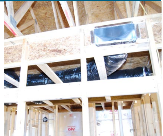
Artistic installs ducts in conditioned space in a duct chase in a dropped hallway ceiling. The air handler for the 9.0 HSPF furnace is also located in conditioned space.
