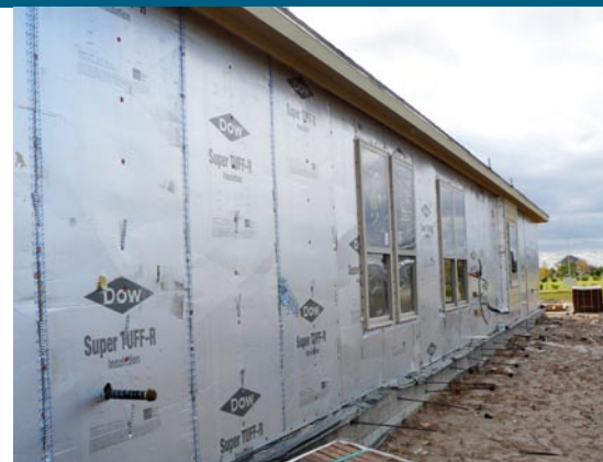
Rigid foam insulating sheathing is taped to provide an air and moisture barrier, a technique recommended by Building America's Building Science Consortium team.
