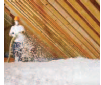
In attic applications, EcoFill Wx blows smooth and fast, providing superior coverage.
