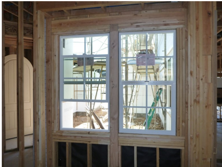
Figure 1. Example of excessive framing at windows (recessed in 2 × 6 wall)
