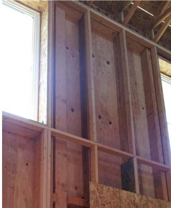
Figure 13. Great room double-stud wall with ¼-in. air gap between interior and exterior framing
