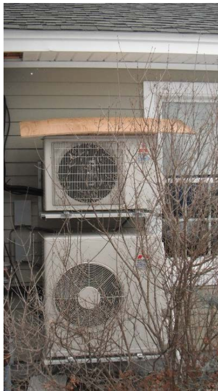
Figure 39. Heat pumps at Site 8. During short-term testing, the lower unit entered defrost mode every 10 minutes; CARB suspects this was largely a result of defrost water from the upper unit refreezing on the lower unit
