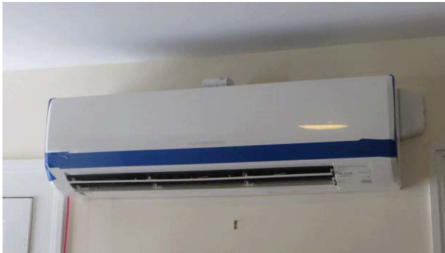
Figure 7. FE18 with return leakage pathway taped
