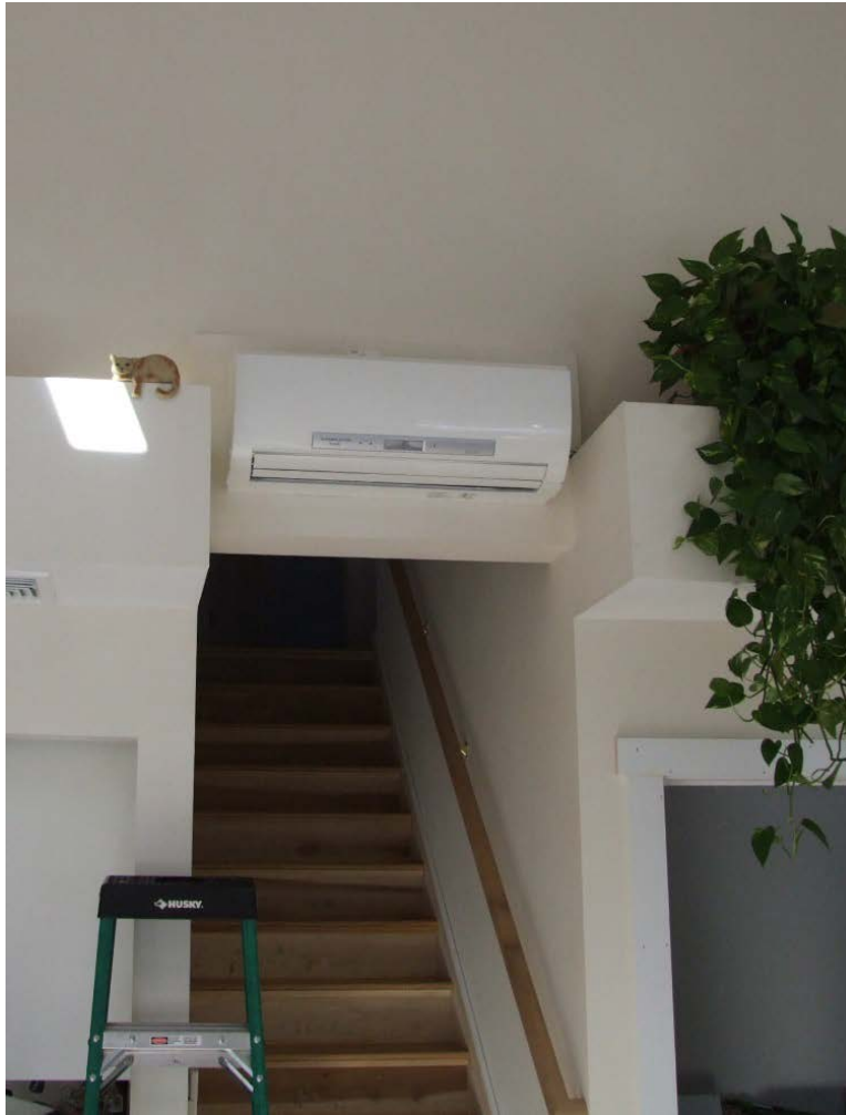
Figure 36. The heat pump at Site 2 was located above a stairway in an area with a vaulted ceiling. This location may have led to relatively high return air temperatures
