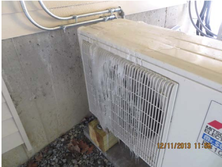
Figure 38. Snow melting from deck above causes icing and excessive defrost on this heat pump (not one of the units monitored for this study)
