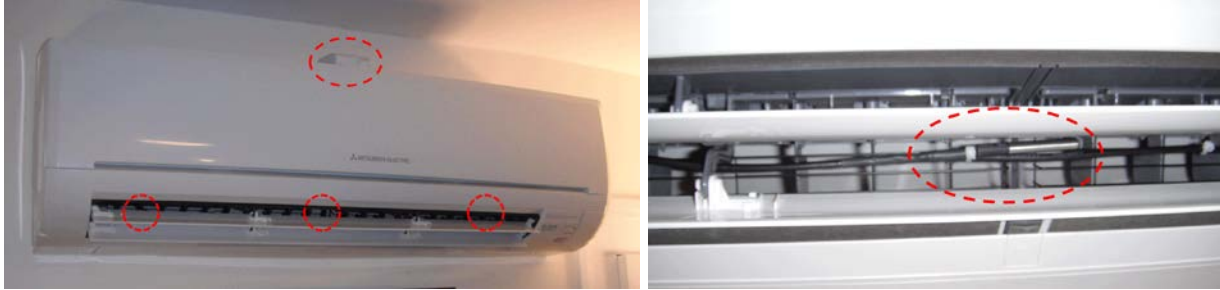
Figure 1. At left, supply and return temperature sensor locations. The right image shows a close-up of the supply temperature sensor
