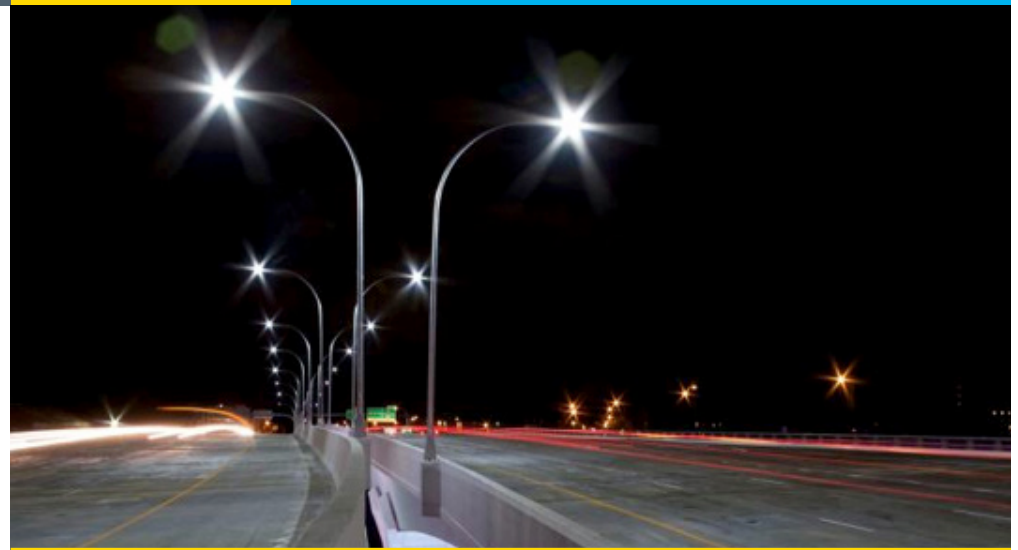
LED luminaires on the I-35W Bridge
