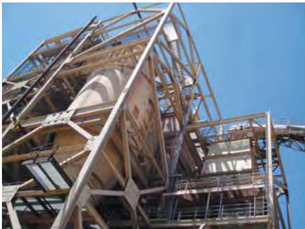
Rio Bravo Power Station
