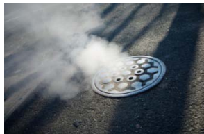
Leaking Steam Traps
