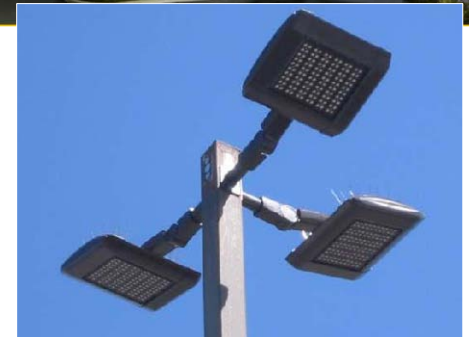
Close up view of new LED luminaires atop an existing light pole.
