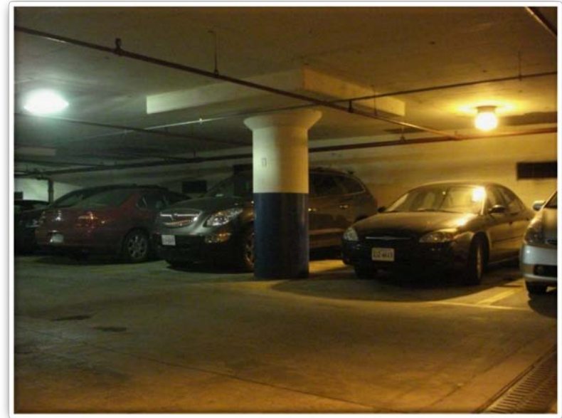
LED on left/HPS on right Department of Labor Headquarters, Washington, D.C.
