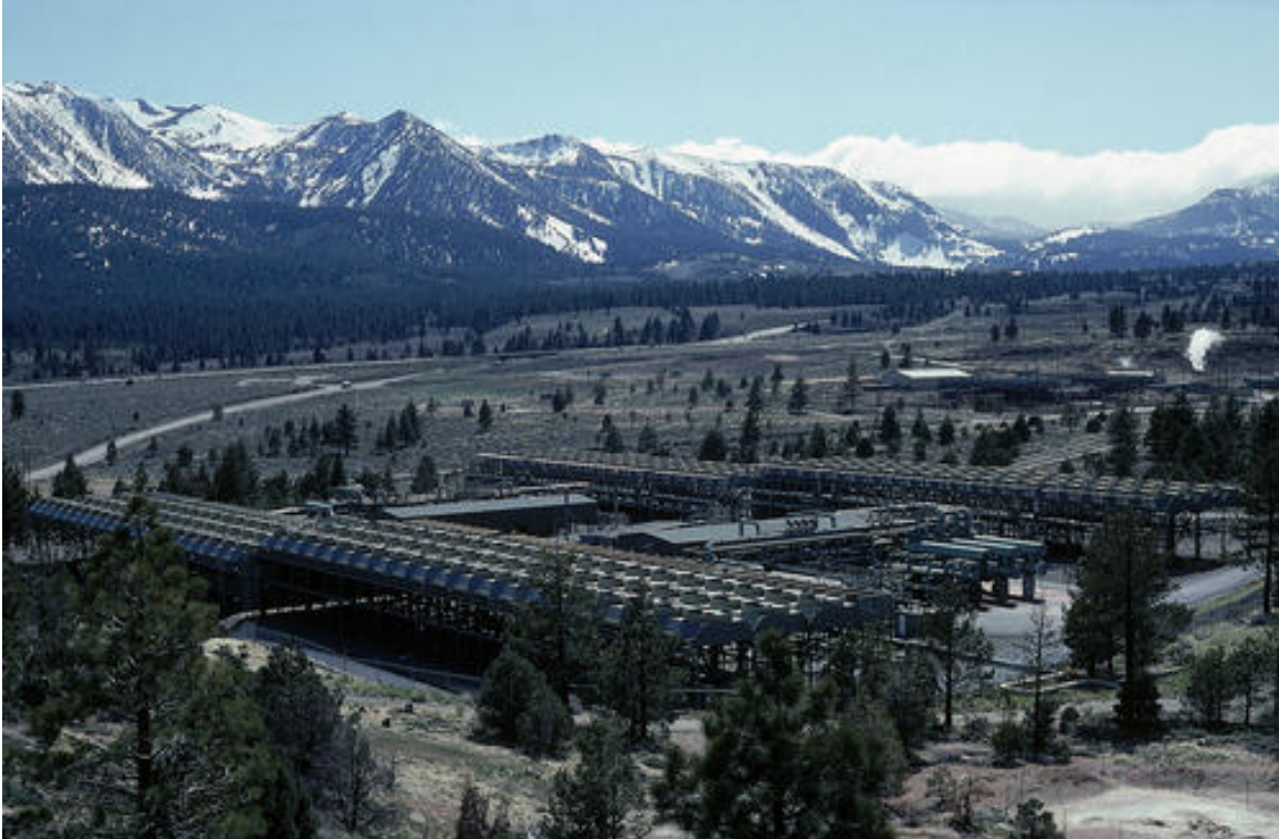
Figure 3.12 – At the Mammoth Geothermal plant, three air-cooled binary units generate a total of 28 megawatts of electricity and release essentially no emissions to the atmosphere or land surface.
