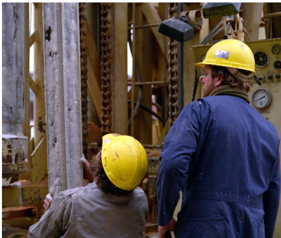
Figure 1.2 - A geothermal heat pump system is being installed in a newly renovated building on the Georgia Tech Campus before the 1996 Summer Olympic Games in Atlanta.
