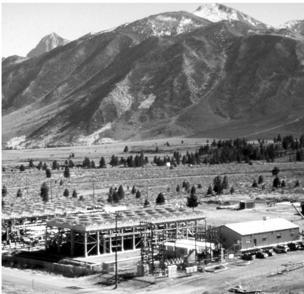
Mammoth Lakes Power Plant, California.
