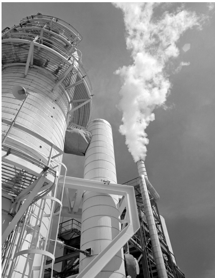
The Leathers geothermal power plant, located in the Salton Sea geothermal resource area. Photo by Warren Gretz, NREL.
