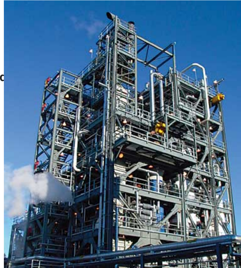
Nikiski AK FT Plant
