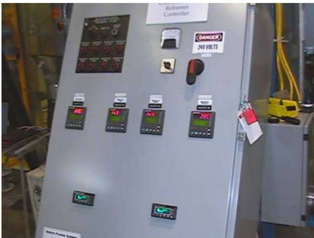
Figure 7: Photographs of the pilot scale reformer and its control panel
