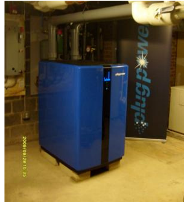
High temperature system at Union College demonstration
