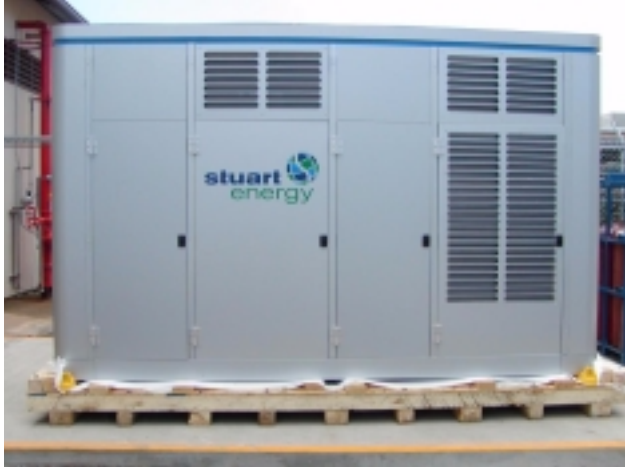
Figure 3. Stuart Energy Systems Electrolyzer at the FCTF
