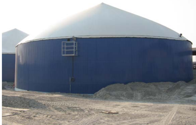
Figure 1. One of two state-of-the-art anaerobic digester tanks where the biogas will be produced. Each tank has an 850,000 gallon capacity and will produce enough biogas to operate a 710 kW engine to generate renewable electrical power.
