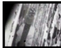
A faulty sootblower is revealed to have lost its head
