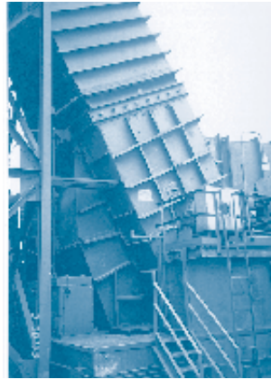
Variable frequency drive and other modifications boost efficiency of BOF fan system by 50%.
