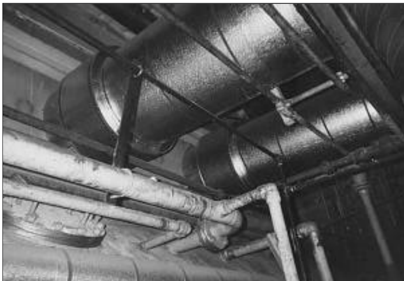
Low-pressure Steam Line
