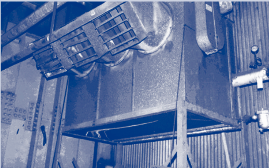
Steam Heater for the Tin Mill (Project 6)
