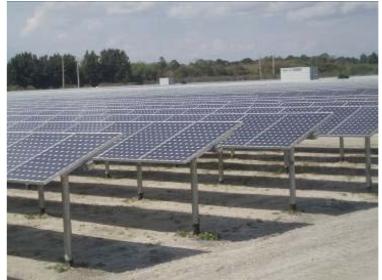
Caption: FPL's 10 MW Cape Kennedy PV Plant
