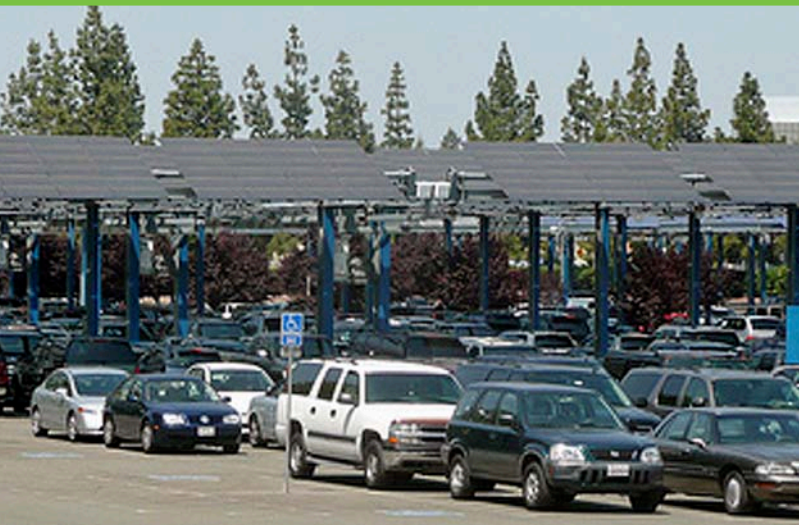
A 540-kW PV system at the California State Exposition Fairgrounds produces power while providing shade for parked cars. Photo from Sacramento Municipal Utility District (SMUD), NREL/PIX 19474
