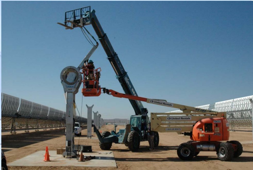
Drive Pylon Commissioning
