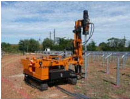
Figure 8: Low levels of automation for solar field installations are just beginning to be developed. http://www.philadelphia-solar.eu/philadelphia_solar_gallery.html
