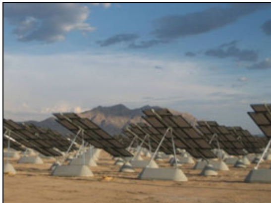
Figure 3. Nellis AFB PV Installation
