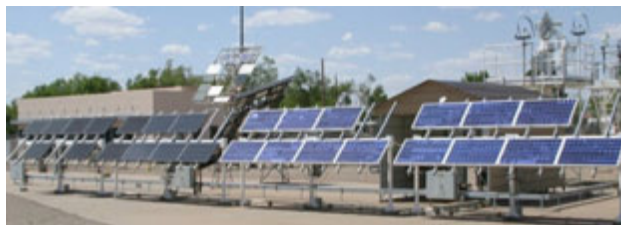
Fig. 1. Systems installed at SNL's PV Systems Optimization Laboratory
