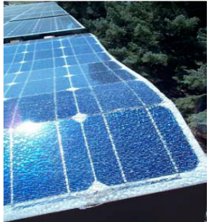
Glass breakage can present high-voltage safety problems
