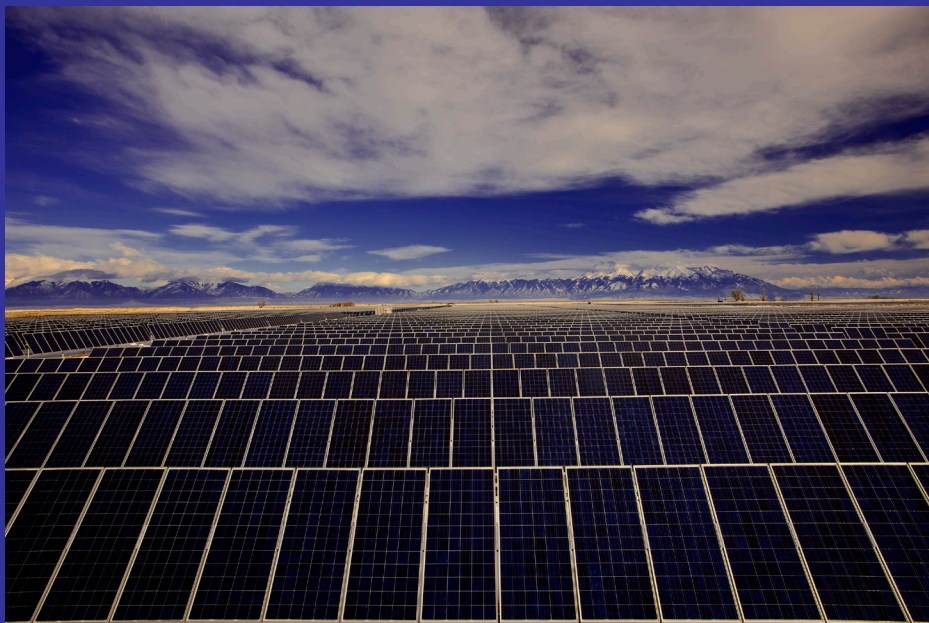
8 MW Solar Field, Alamosa, Colorado, USA: Photo courtesy of SunEdison and Zinn Photography
