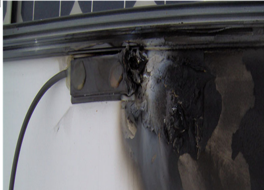
Arcing – Junction Box
