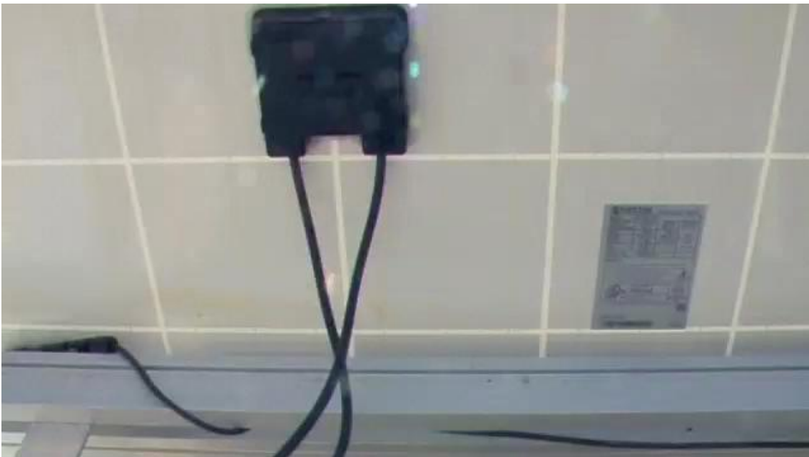
Single Module Arc Test
