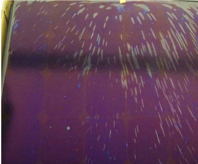
Photo of module with delaminating AR coating
