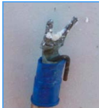
Corroded signal connections
