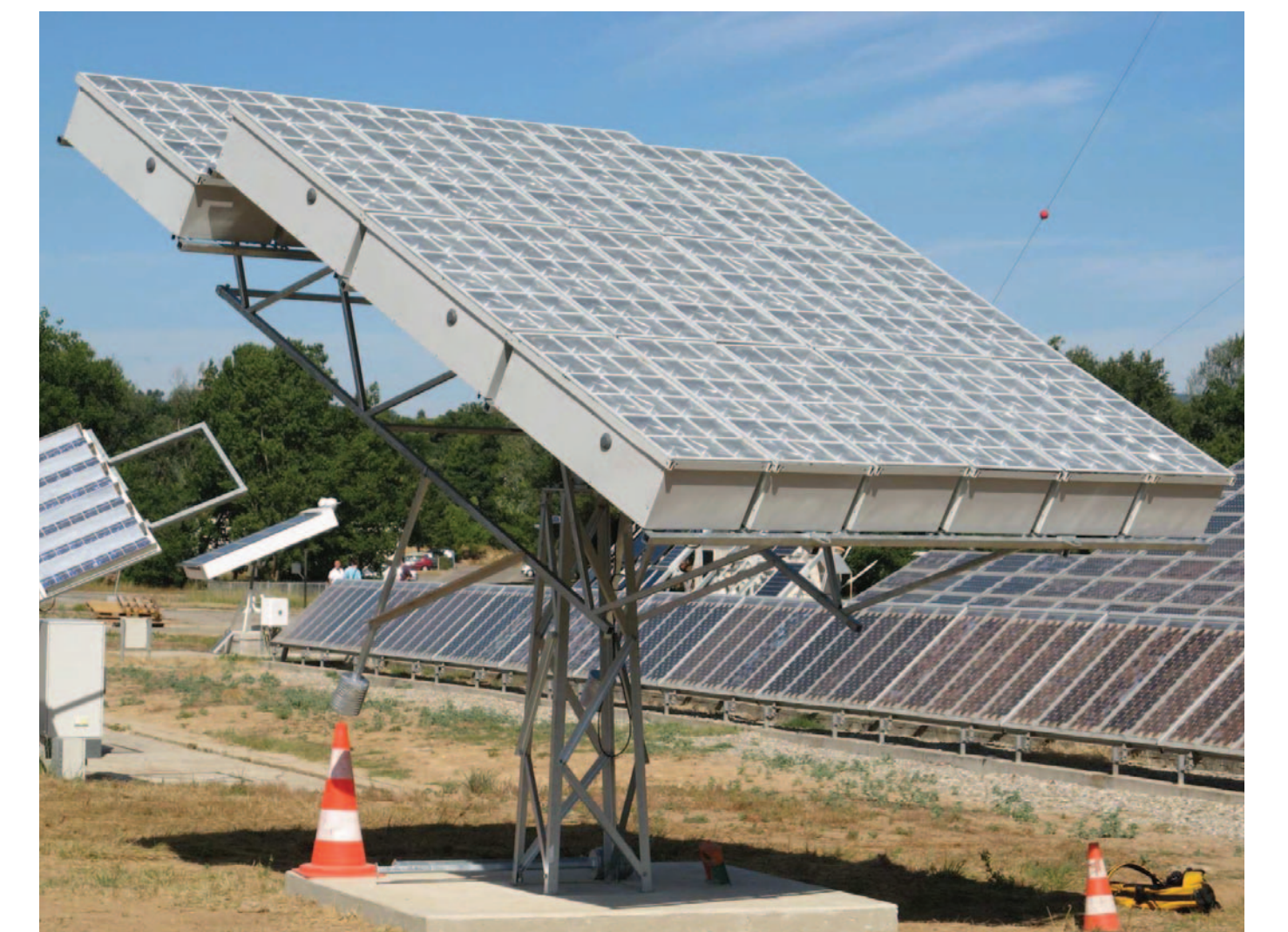
Tracker installed in CEA-Cadarache (south of France)
