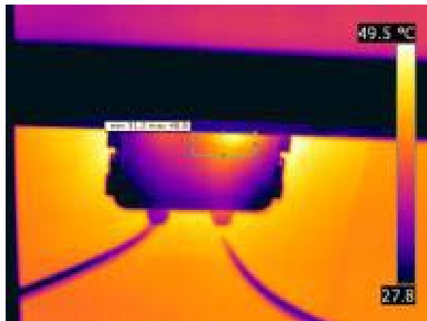
Figure 1: IR image of a junction box with high contact resistance.
