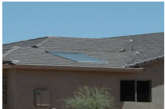
Fig. 2. In 2006, Sandia helped the solar industry obtain SRCC certification for a roof-integrated solar hot water system.
