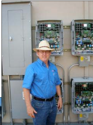
Inverter installation at SAS Forest City
