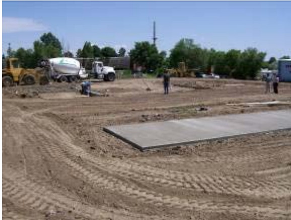
Lakewood Test Site – 2 mini-collectors (phase 1 now complete)
