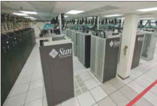
Sandia National Laboratories/ New Mexico High Performance Computing Water Reduction and Energy Efficient Cooling
