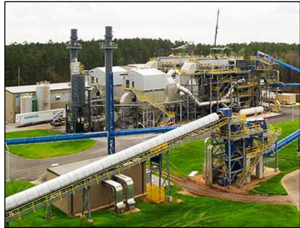
Savannah River Site's Biomass Cogeneration Facility
