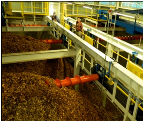
ORNL's New Biomass Steam Plant
