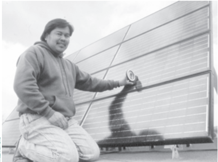
KEVIN BEGAY CHECKING THE INCLINATION OF PV PANELS FOR THE HOPI SOLAR ELECTRIC ENTERPRISE PROJECT
