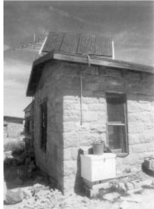
A PV SYSTEM ON THE HOPI RESERVATION WITH 4 MODULES AND AN EXTERIOR BATTERY BANK INSTALLED BY NATIVE SUN.
