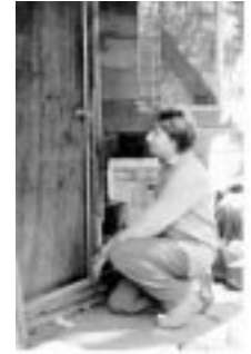
HOOPA TRIBAL MEMBER WEATHERSTRIPPING THE FRONT DOOR OF A TRIBAL HOME. FROM CALIFORNIA ENERGY EXTENSION SERVICE, 1992.
