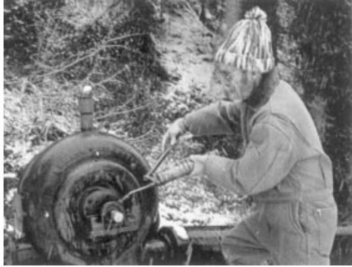
A MICRO-HYDRO SYSTEM OWNER PERFORMS THE WEEKLY GREASING OF HIS HYDRO TURBINE (PHOTO: FRONTIER ENERGY, STATE OF ALASKA, 1984).
