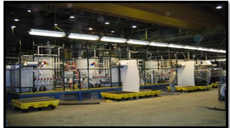
Plastics Recovery Facility
