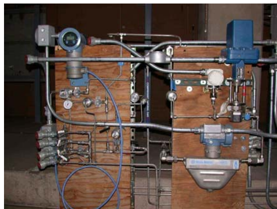
Figure 2. 100% hydrogen, CNG, and 15, 20, 30, and 50% blended HCNG (by volume) prototype dispenser brassboard design.
