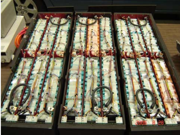
Figure 2. Lithium Ion Battery Pack Used in EnergyCS Conversion of a Toyota Prius
