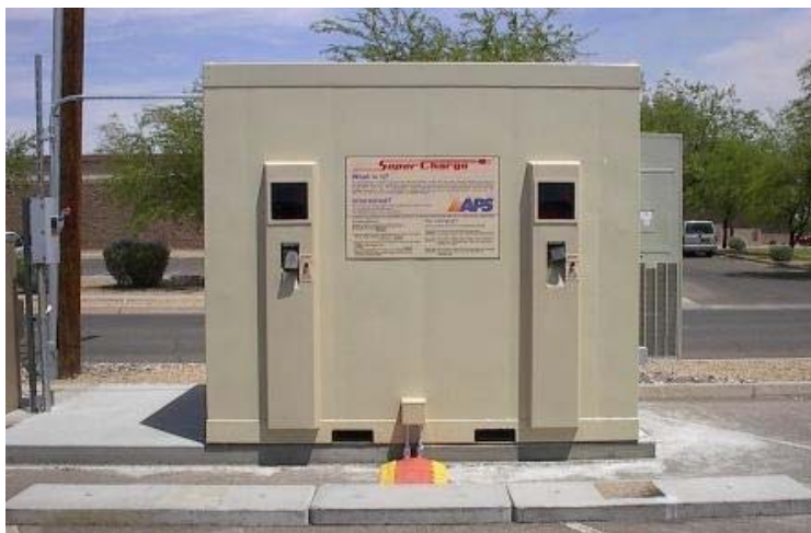
Figure 1. Luke Air Force Base SuperCharge Station
