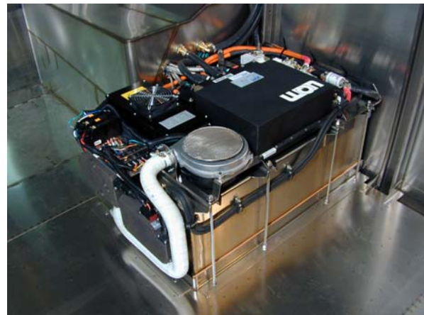
Figure 9. Installed propulsion system
