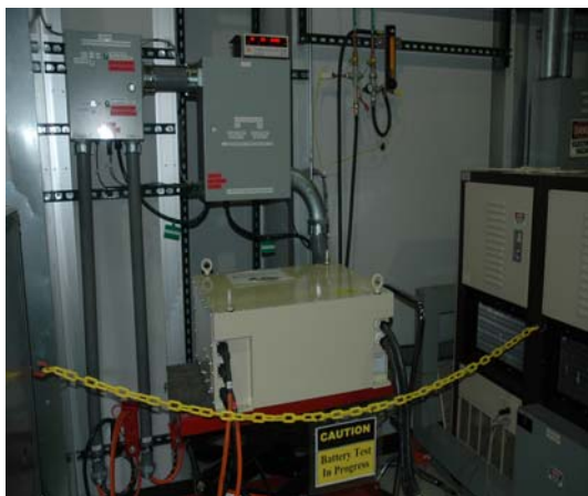
Figure 6. External Fuse Box, Contactor Box, Cooling Water Feed to the Battery
