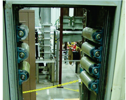
Figure 7. Free-roller systems as installed between oxidation ovens.
