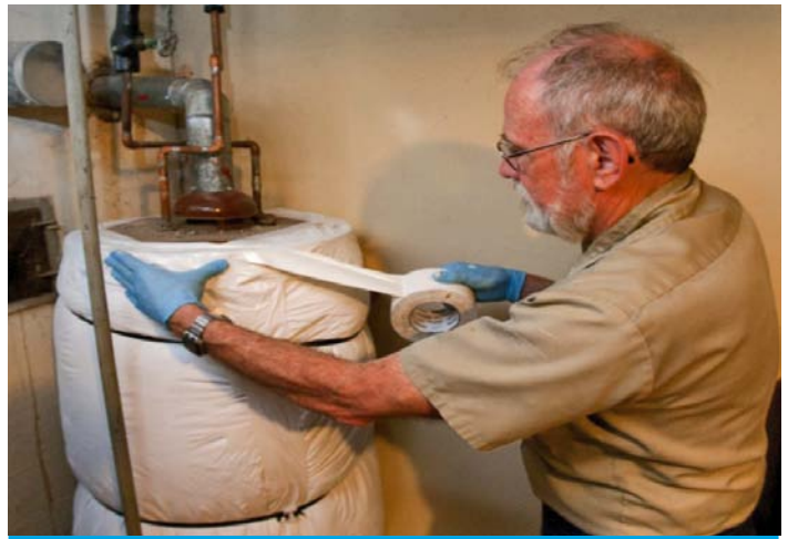
Volunteer David Legg insulates a water heater. Photo by Chris Cone Photography for PWC
