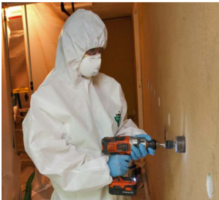
Volunteer London Huenefeld drills holes for wall insulation installation. Photo by Chris Cone Photography for PWC
