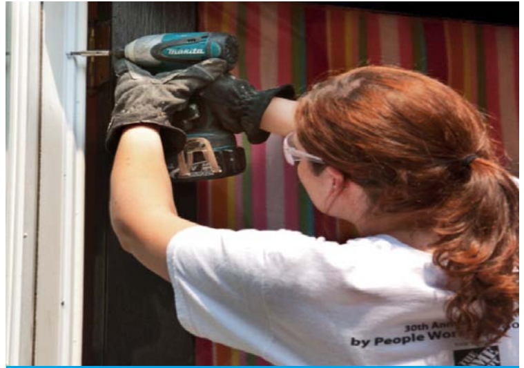
Weatherization volunteer London Huenefeld works on air sealing a door. Photo by Chris Cone Photography for PWC
