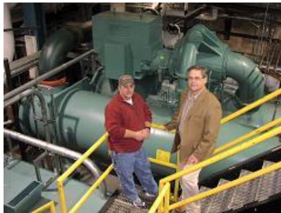
Bruce Stultz (right) with Central Plant Manager Mike Penyak and a new chiller in a DGS facility.
