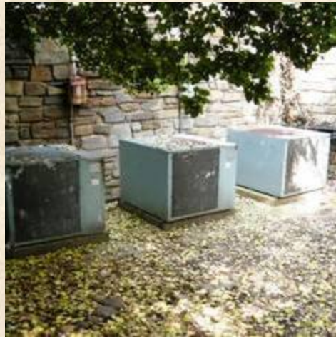
Old heat pumps
