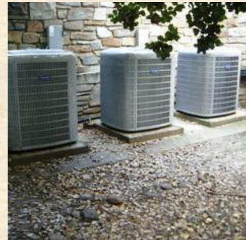
New heat pumps
